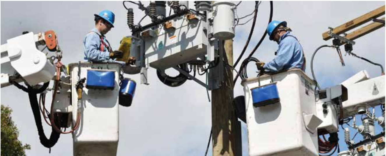
Multiple forces are reshaping the U.S. electrical grid, creating unprecedented opportunities to operate properties efficiently. (Photo: Con Edison)
